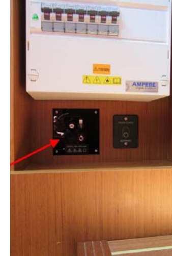
Indoor socket circuit breaker Location: Companionway
