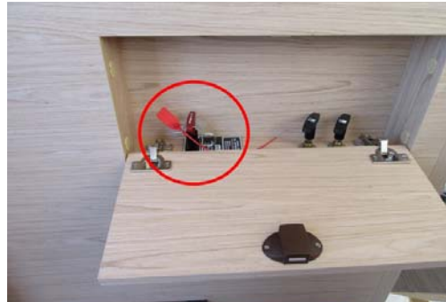
Ref 2: Remote pull switches Location: Wheelhouse
