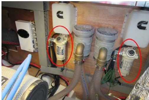
Location: Engine compartment
