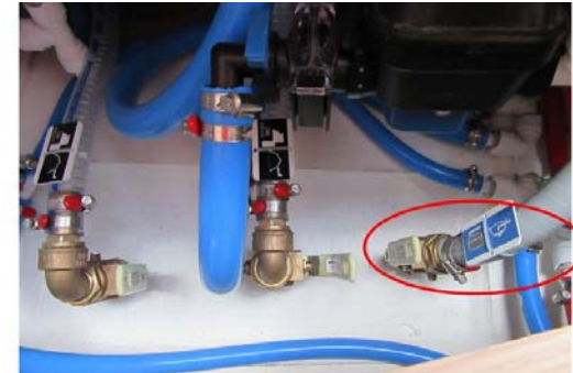
Waste water drain valve to the sea
