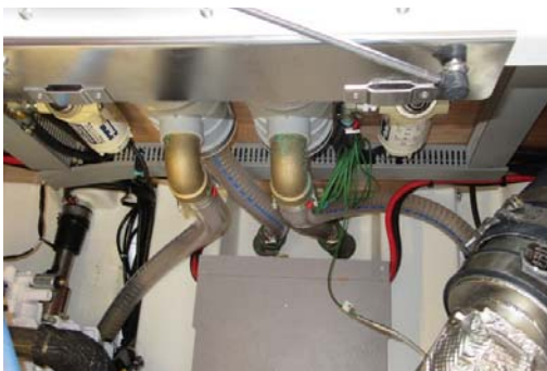
Engine water intake valve Location: Engine compartment
