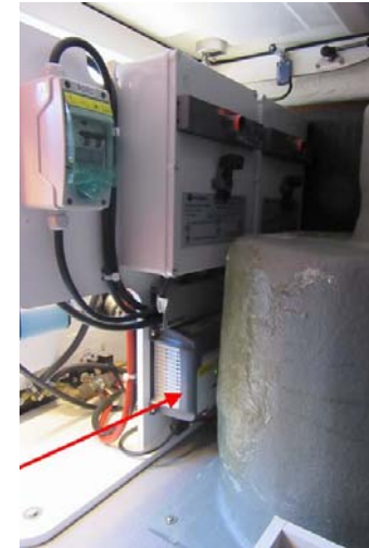
Generator battery charger (12V circuit)
