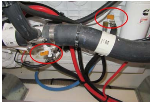
Port engine/demister cooling system supply valve
