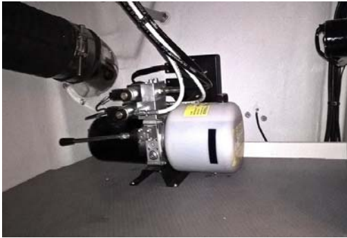
Location: Cockpit locker
