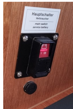
Servis batteries red main breaker
